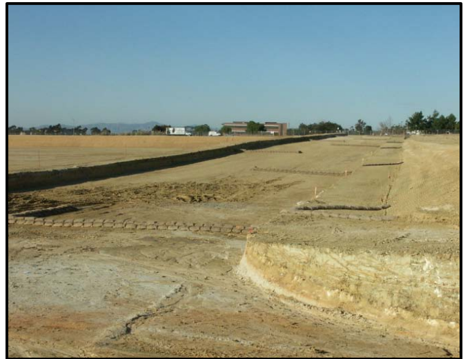
Rough Cut Street Control along dirt road - credit to Urban Drainage and Flood Control District
