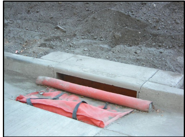
Storm Drain Inlet Protection
