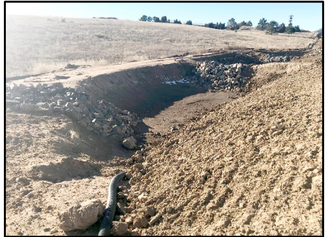
Sediment Trap downstream of rock check dams
